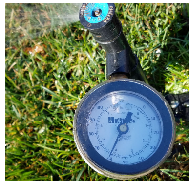
Water pressure can be tested at the valve or the sprinkler head.
