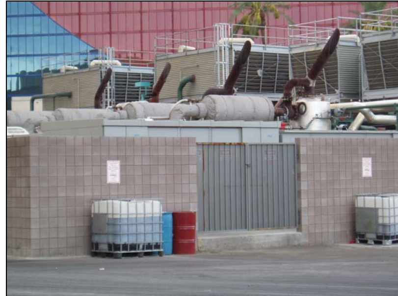
Ipanema CHP Station (~3.2 MW) Rio All-Suites Hotel & Casino, Las Vegas
