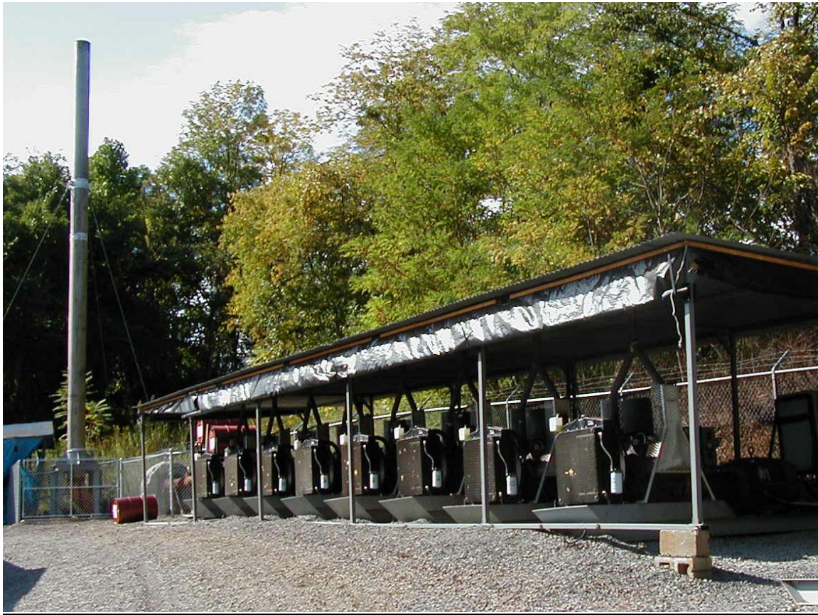
675 kW Synchronous Skid-Mounted Generator sets at Nelms No. 1 Mine, Ohio (Photo courtesy Northwest Fuel Development, Inc. and U.S. DOE)
