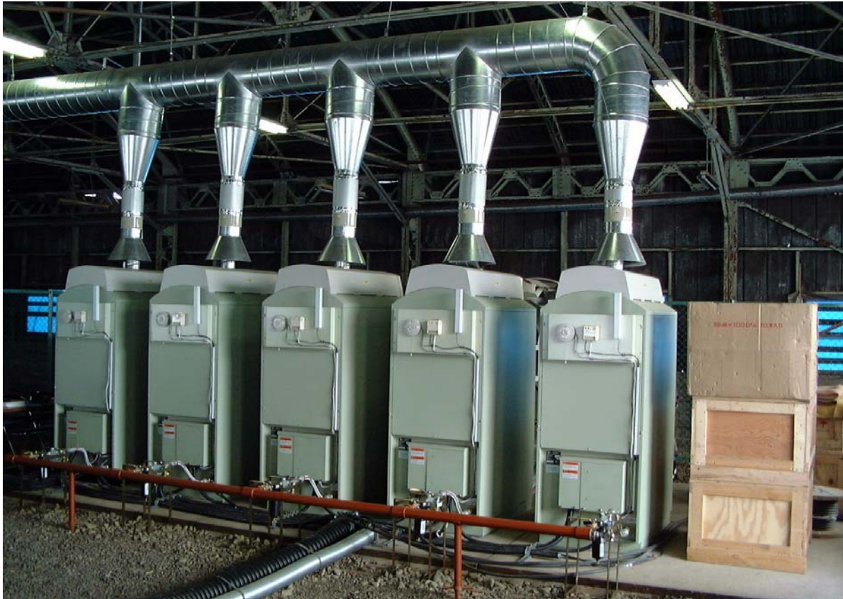
Five Capstones Micro Turbines Operating at abandoned Akabira Mine in Japan (Photo courtesy of Raven Ridge Resources)
