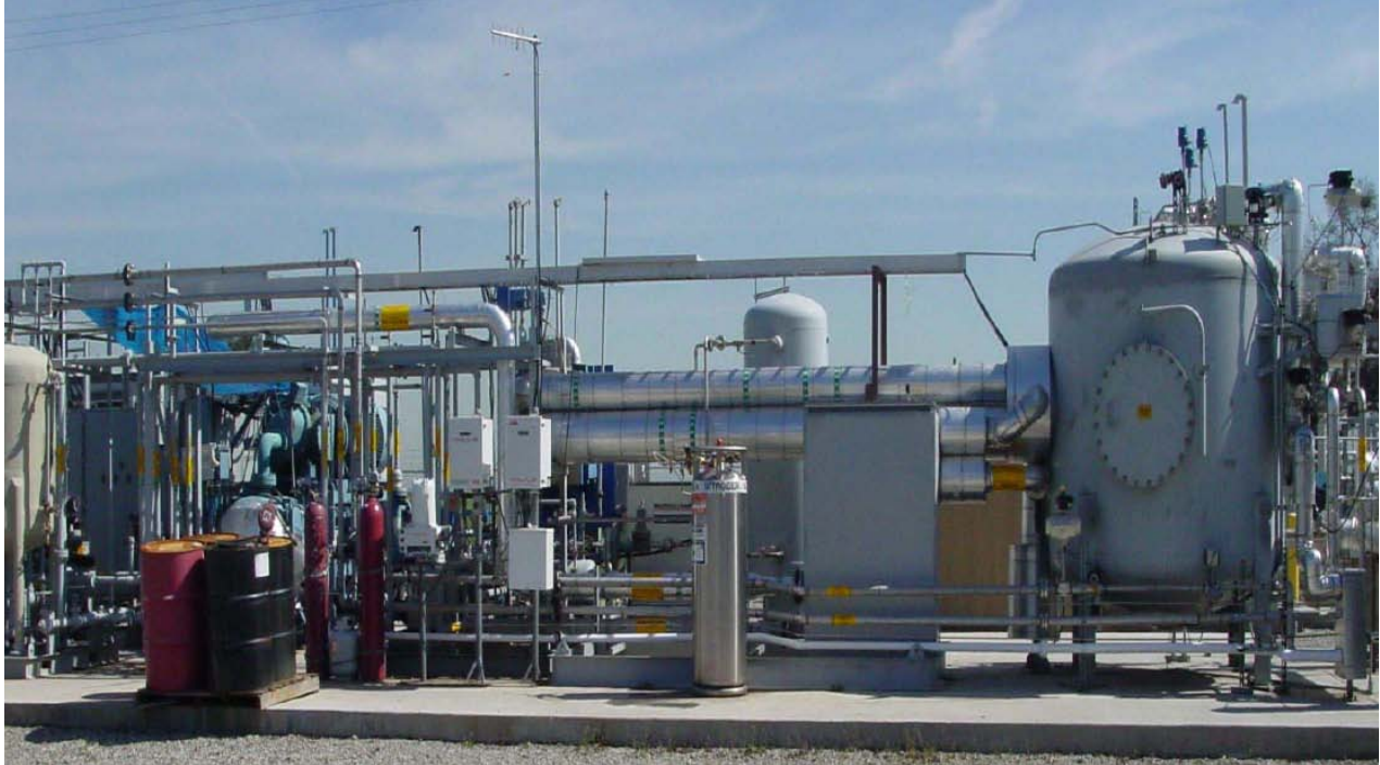
Example of a small scale LNG plant (built by a predecessor company to Prometheus Energy)
