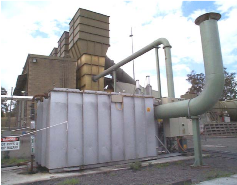
VOCSIDIZER Installation - Appin Colliery (Photo courtesy of BHP Billiton)
