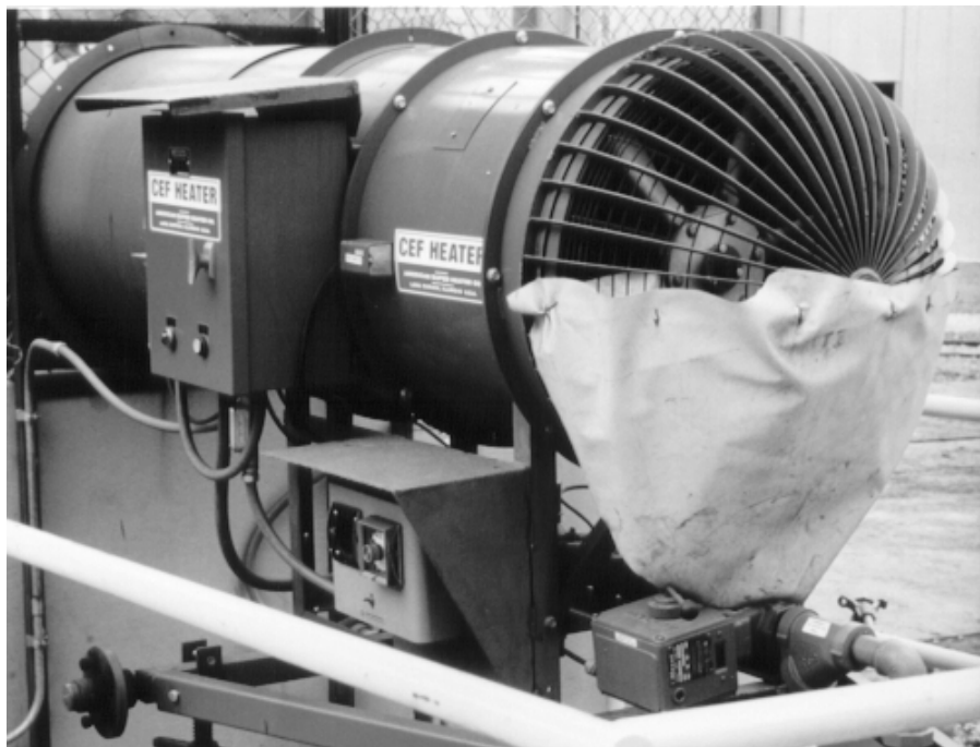
Coal mine methane-fueled heater at one of the Jim Walter Resources mines in Alabama (Photo courtesy of Jim Walter Resources, Inc.)
