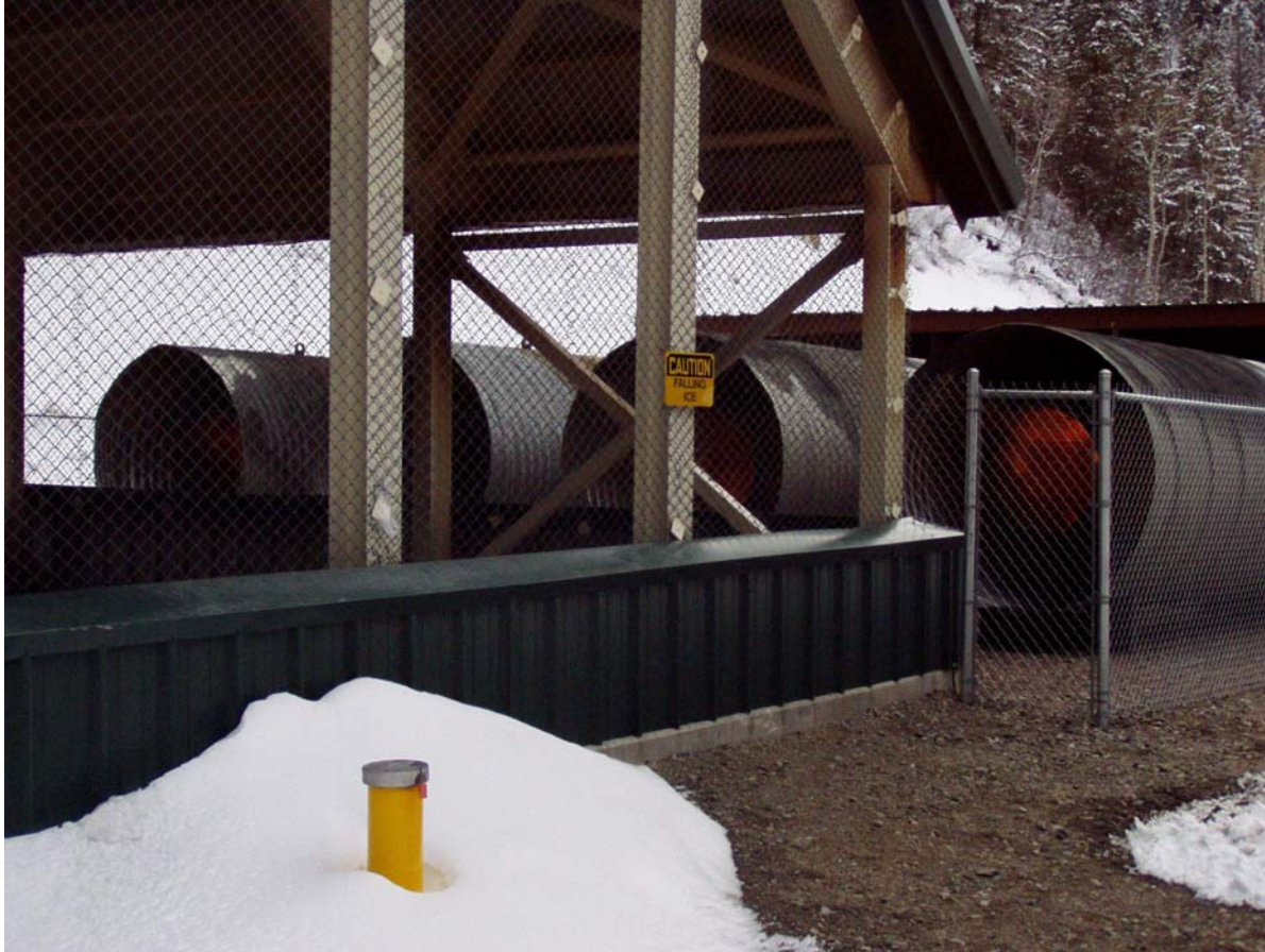
Coal mine methane-fueled heaters at a mine in the Rocky Mountains (Photo courtesy of Raven Ridge Resources, Incorporated)
