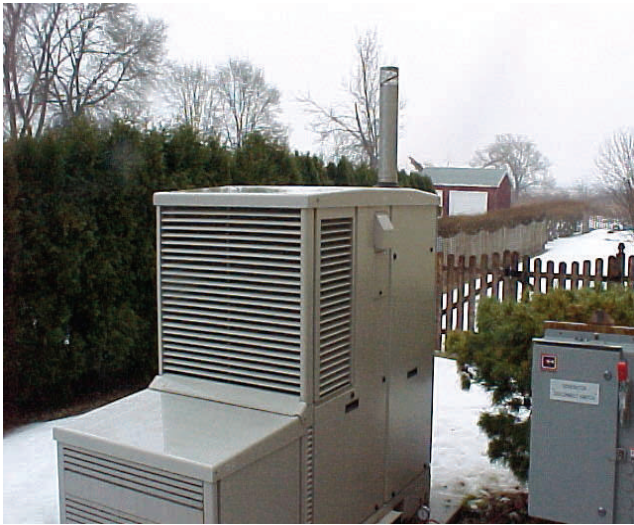
Plug Power Fuel Cell
