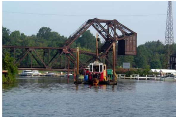
Cutterhead suction dredge removing contaminated sediments from the Ashtabula River turning basin
