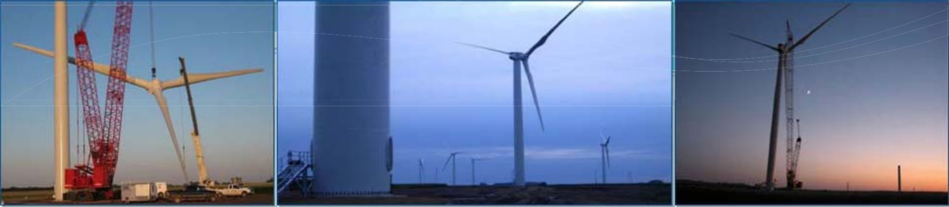
National Wind Project, Jeffers, MN
