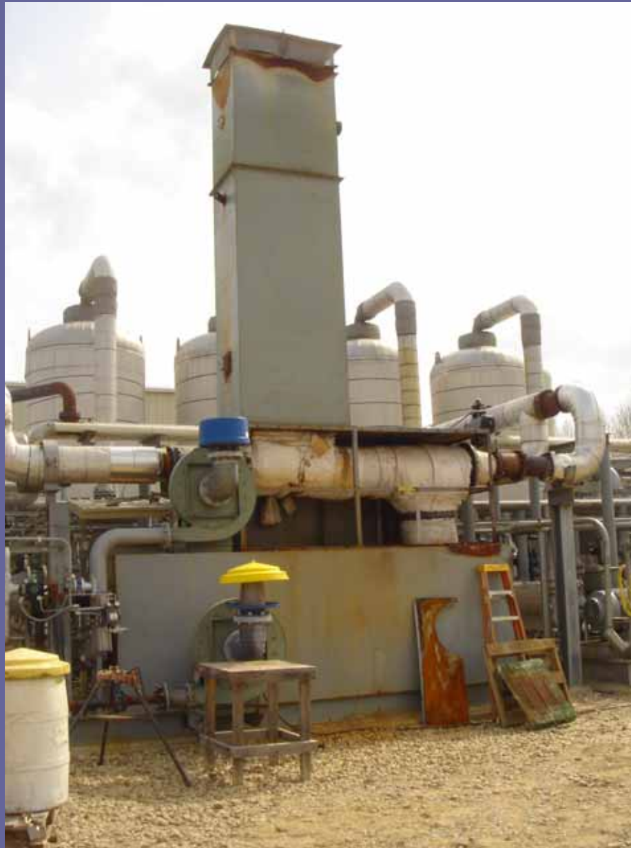
McComas Thermal Oxidizer. High temperatures destroy VOC's.
