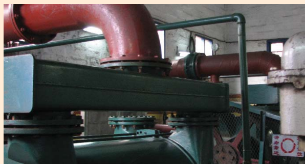
Pumping station at a mine under study in China. The station extracts methane from the underground coal seam in advance of and during mining.
