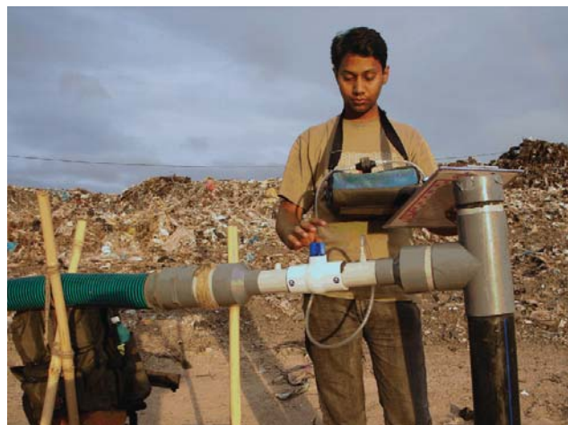
Extraction well monitoring at the Uruli Devachi Landfill in Pune, India.
