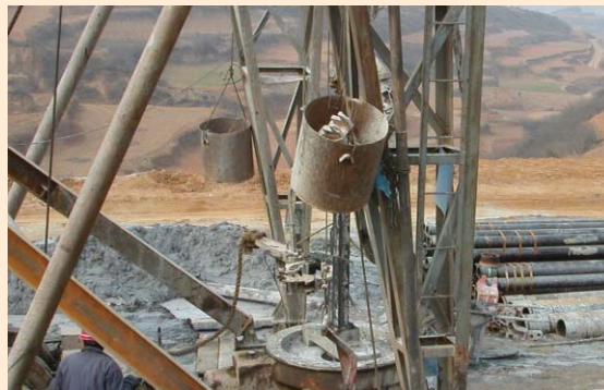
Construction of the world's largest CMM-generated power project (120 MW capacity) at Sihe Mine, Jincheng, Shanxi Province, China.
