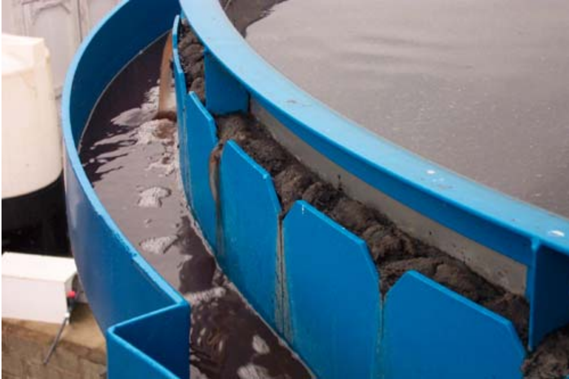
Figure 4-3. Floating solids block effluent weir.
