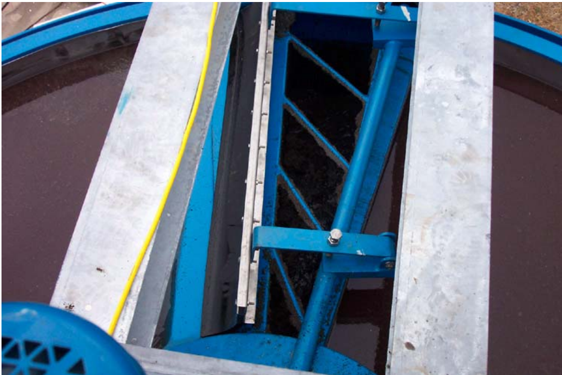
Figure 2-3. Floating solids skimmer box.
