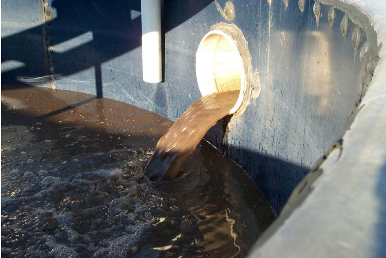
Figure 3-1. Mixing tank receiving wastewater influent.
