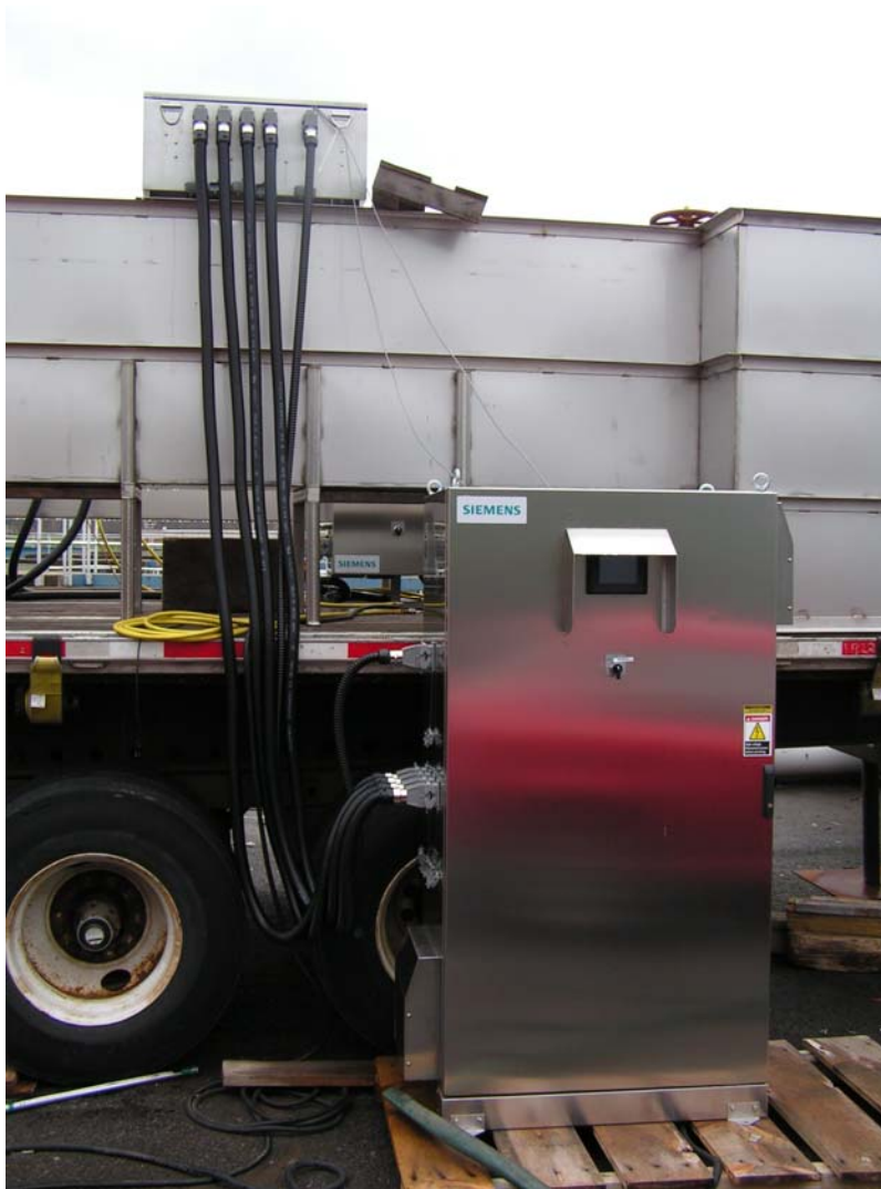
Figure 3-5. Photo of unit cables and power panel.
