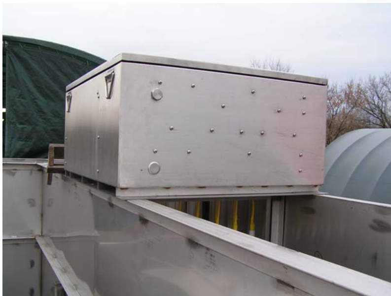
Figure 3-4. Photos of V-40R-A150 reactor installed in channel.
