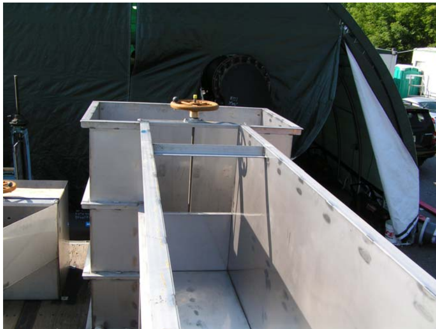
Figure 3-3. Influent stilling plate and effluent weir gate for the Siemens H-4XE-HO (2W-1B-1C) UV unit test channel.
