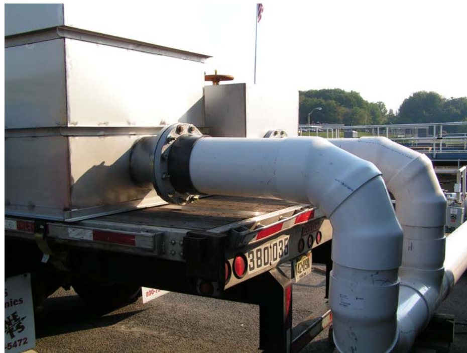
Figure 3-2. Influent (top) and effluent (bottom) piping configuration for the H-4XE-HO (2W-1B-1C) test unit channel.
