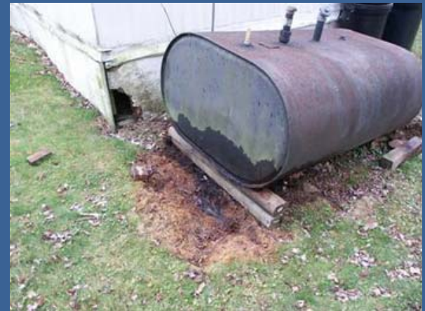
Leaking Oil Tank Responsible for Contaminating Local Water Supplies
