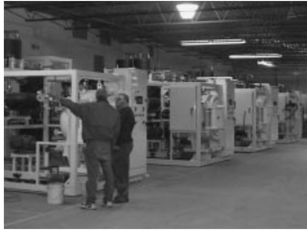
The Micell Technologies Production Facility in Midland, Michigan
