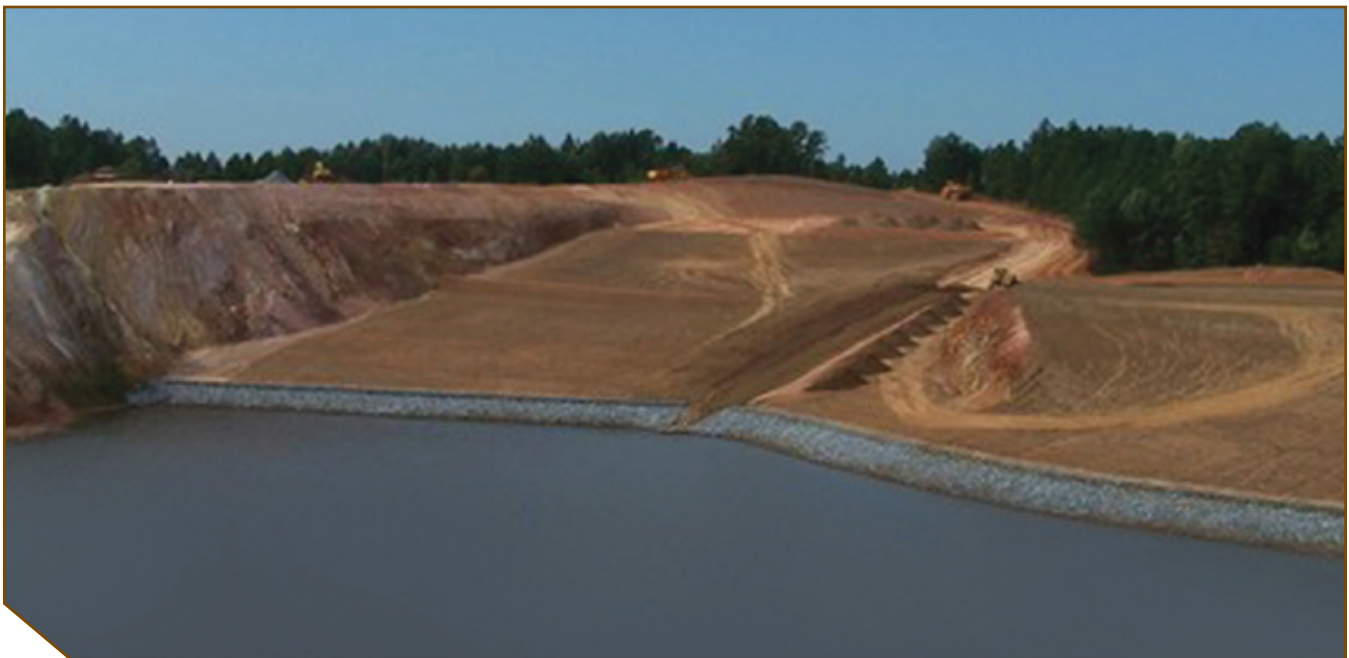
Barite Mine Site. Post-remediation with new cap, retaining wall, and lime-neutralized treatment pit. The remote monitoring system that SCMTSC/INL designed ensures that this treatment pit and cap are working properly and, if necessary, will detect issues so changes can be made, especially in this early stage while the vegetation on the cap takes hold.
