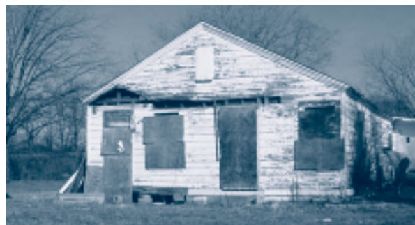
Figure 5 The first structure demolished under Phase 1 of the City of Fort Worth XL Project at 2615 Ennis Avenue.
