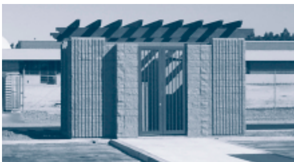
Figure 15 The SUVMS electrical equipment enclosure, which provides power to the SUVMS and EVs charging stations at Vandenberg AFB.
