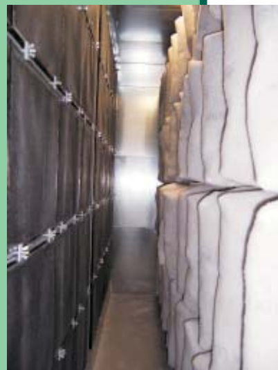
Paint booth carbon adsorption unit
