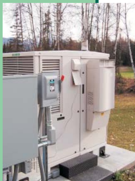
Fuel Cell at Fire Station 3
