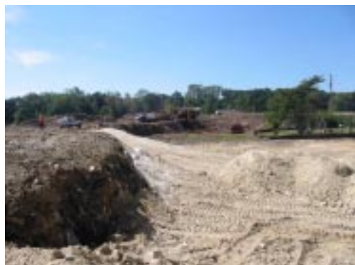
Excavation and consolidation of waste at the Walsh Road Landfill Site (September 2005)
