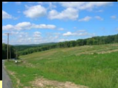
Pictured at left is the completed cap on the south/southwestern slope of the Eastern Diversified Superfund Site, September 2008.
