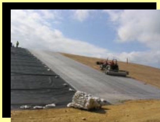
Tractor laying out the geosynthetic and clay liner over the soil sub-base in October 2007.
