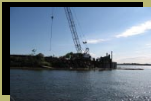
Sheet pile wall being installed along the Delaware River at the Metal Bank Superfund site.
