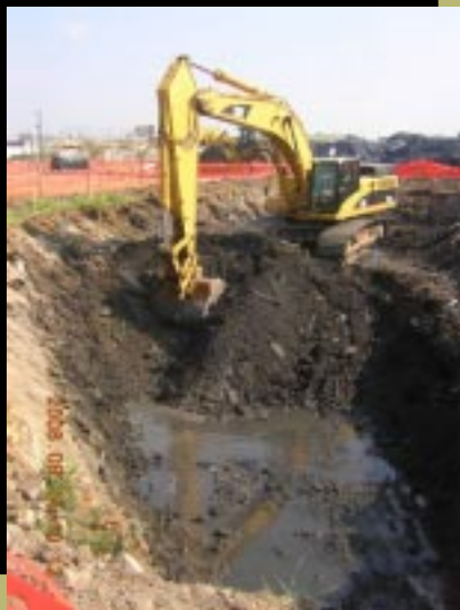
Excavation of PCB-contaminated soils from an inland area of the Metal Bank Superfund Site
