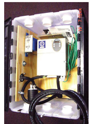
VFD mounted in box
