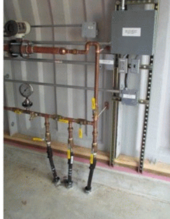
View of piping system inside instrument building.
