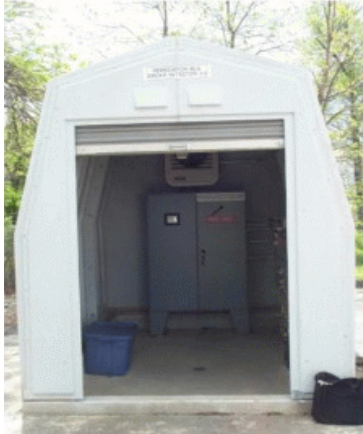
Shed containing instrument panel and piping.
