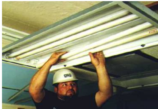
Typical Fluorescent Lamp Fixture. (Townsend 2004)
