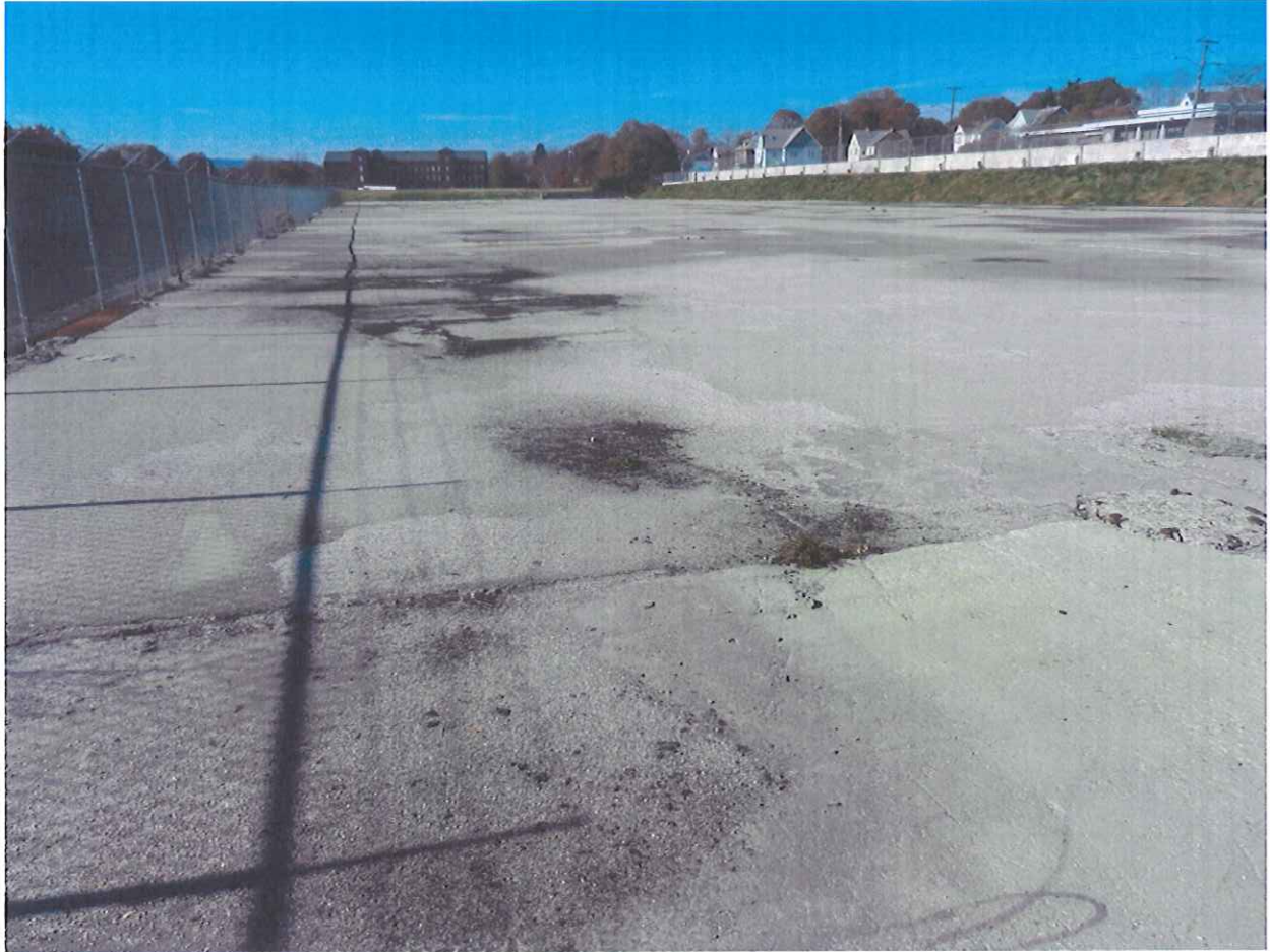
40s Other Ground Covering Feature Area (left) and Slab Area (right) – Looking West 11/9/11
