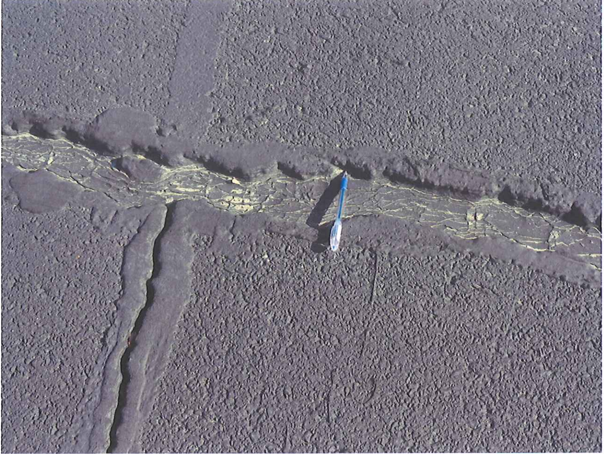
20s Building Demolition Barrier Area #1 Typical Crack Sealed in 2009 11/9/11
