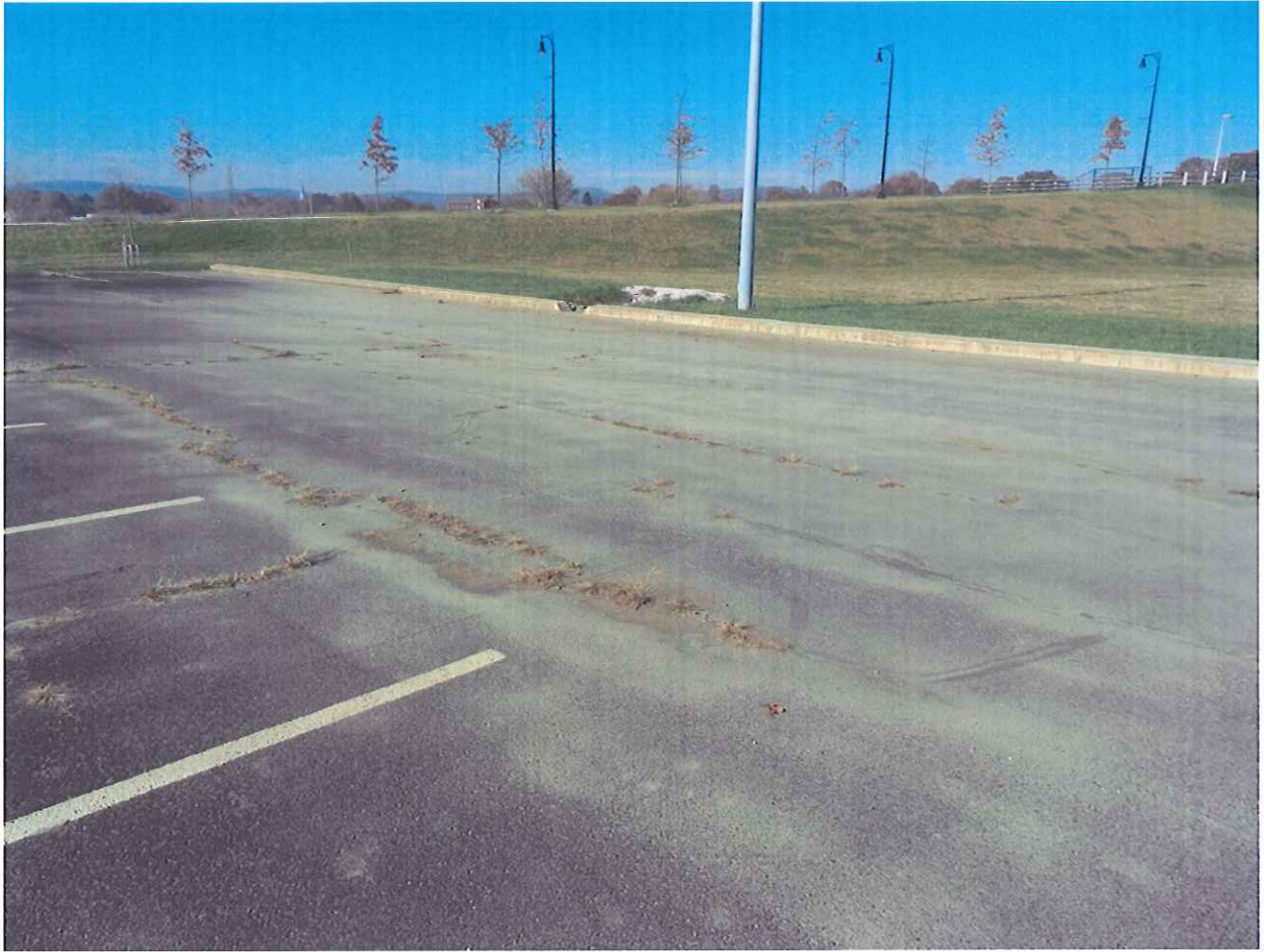
20s Building Demolition Barrier Area #1 Sign of Restricted Drainage 11/9/11
