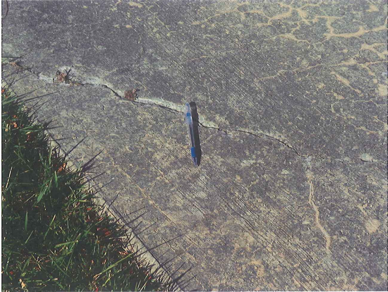
20s Building Demolition Barrier Area #2 Typical Crack 11/9/11
