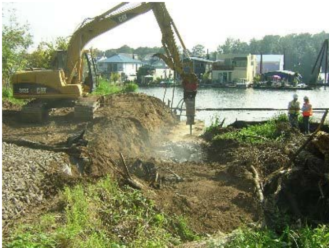
Combined sewer overflow pipe removal at Stephens Creek confluence improves floodplain habitat
