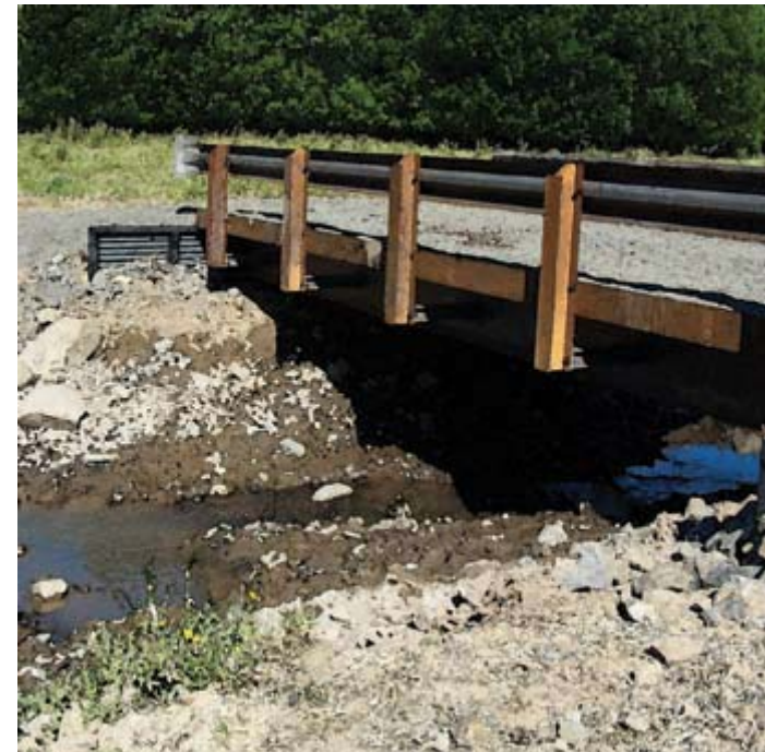
Some restoration plans include culvert removal and bridge construction to allow fish passage
