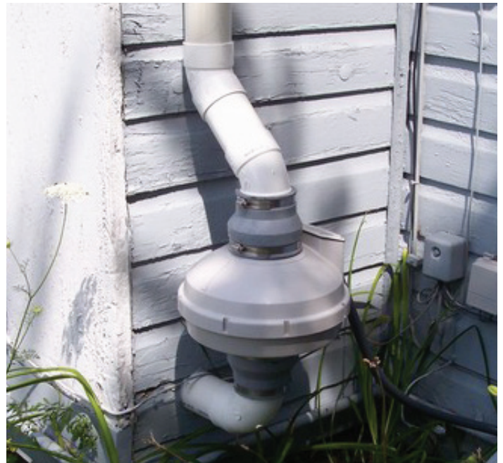
This residential vapor abatement system, which is about the size of a football, could be installed on the outside of a house.
