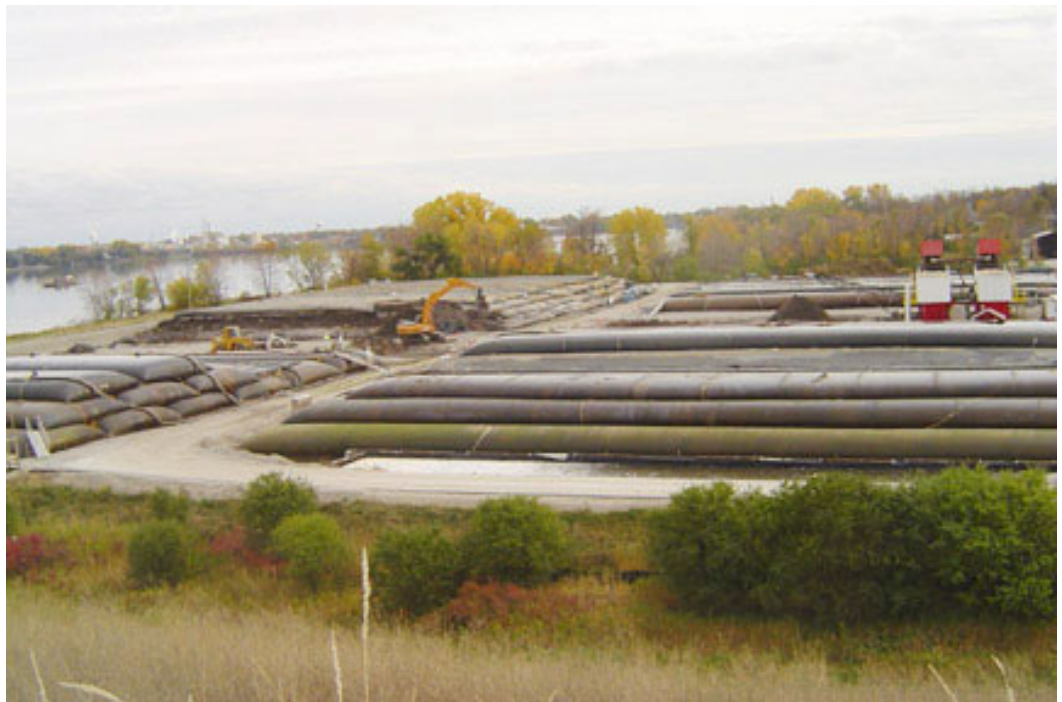
After the sediment is dewatered in geotubes, it is trucked to a landfill.
