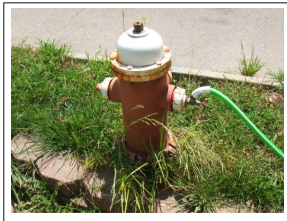
Figure 2-2. Hydrant With Un-metered and Possibly Unauthorized Use
