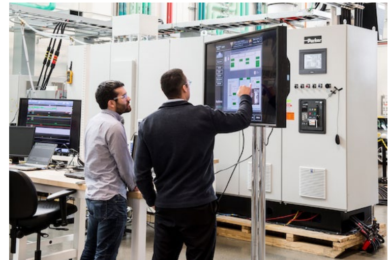
NREL and Raytheon, perform system level testing on the Miramar ZnBr Flow Battery Photo by Dennis Schroeder / NREL 32582
