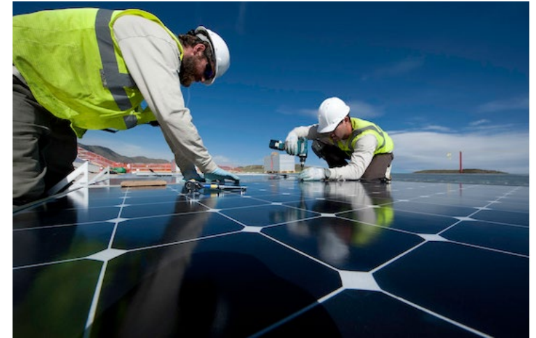
Installation of one of the 3,632 solar modules on NREL's parking garage. The garage can produce up to 1.15 megawatts Photo by Dennis Schroeder / NREL 21487
