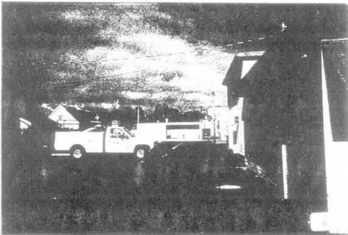
Northwest Transformer, South Harkness Site, Everson, WA
