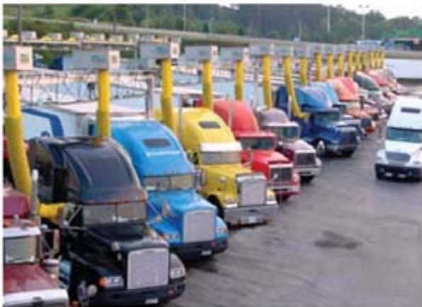
Trucks turn off their engines at a TSE facility and hook up to external air conditioning and power systems...
