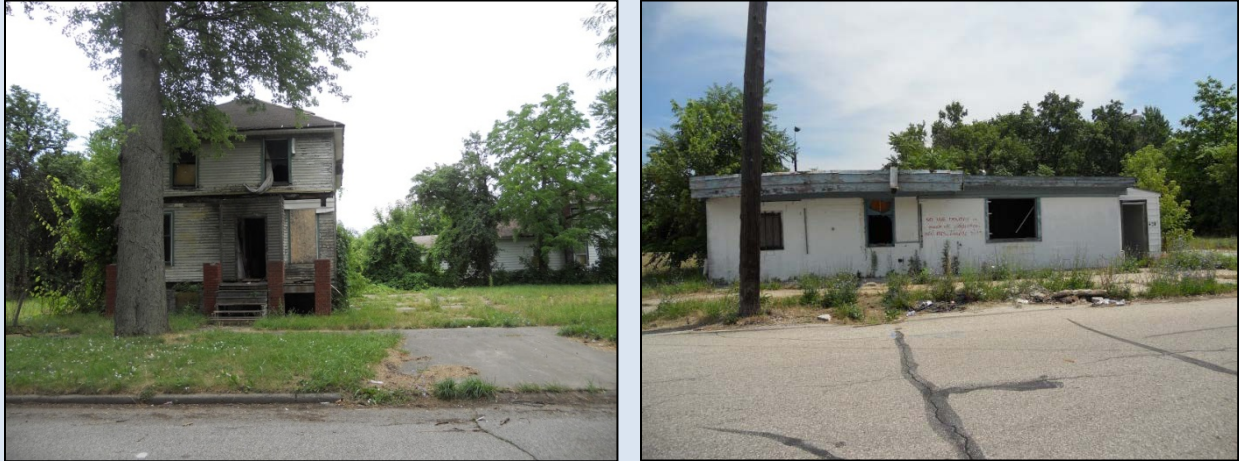
Exhibit 1-4: Vacant and Abandoned Properties in the Green Zone. The Green Zone contains many vacant and abandoned properties that are uninhabitable in their current state and pose a potential risk to public health and safety.
