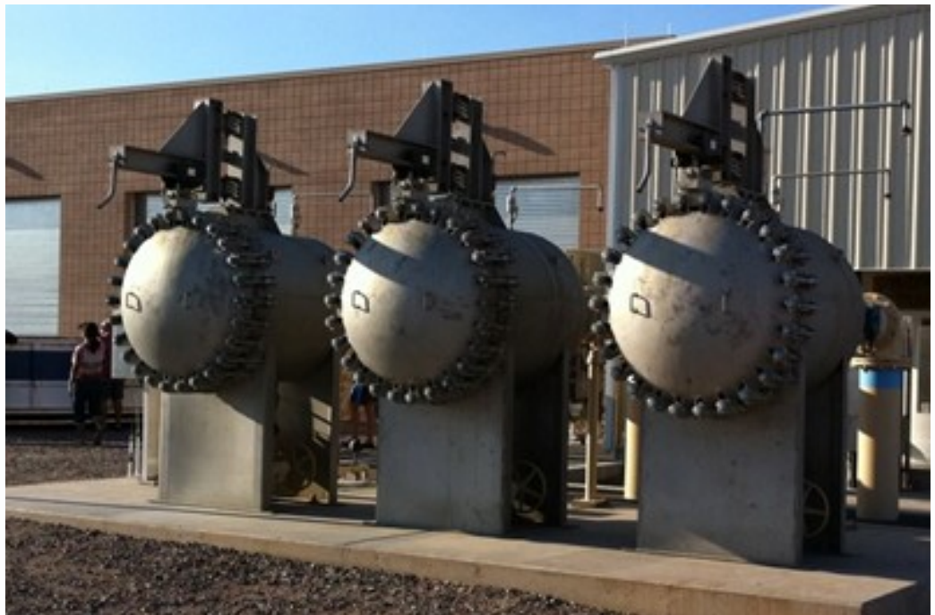
Reverse Osmosis Water Treatment Plant, Gila River Indian Community.
