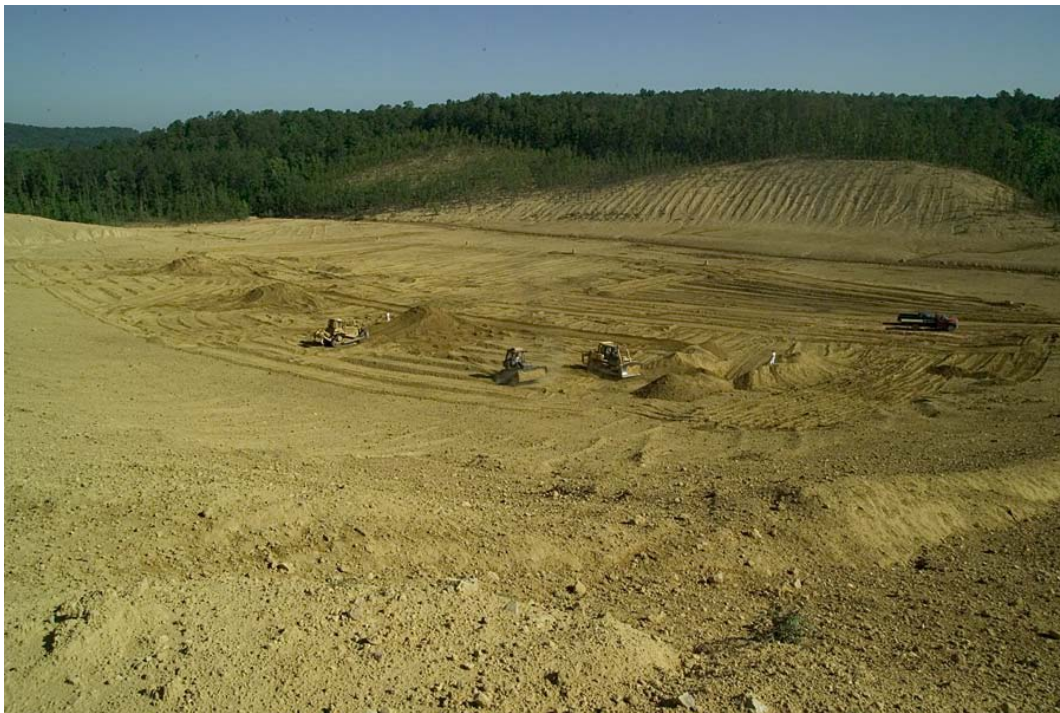
FIGURE IV B-7 OD Unit as Pictured from South to North
