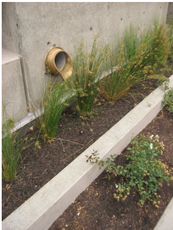
Figure 9. Disconnected downspout discharging to planter box.
