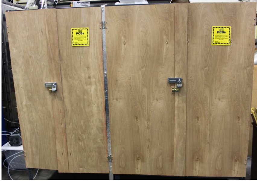
Figure 2.9. Wooden cabinets that housed the plastic cabinets
