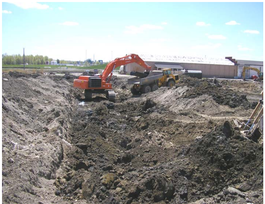
A large excavator does preliminary clearing in the area that will soon become a special landfill. Contaminated sediment from the Ashtabula River will be contained permanently in this landfill.
