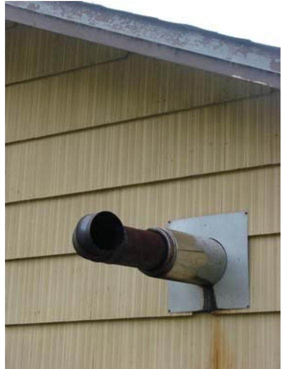
Woodstove stack prior to change out.
