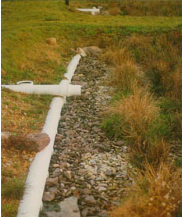
A recently expanded Subsurface Flow constructed wetland system serves the small community of Monterey in Highland Co., Virginia.
