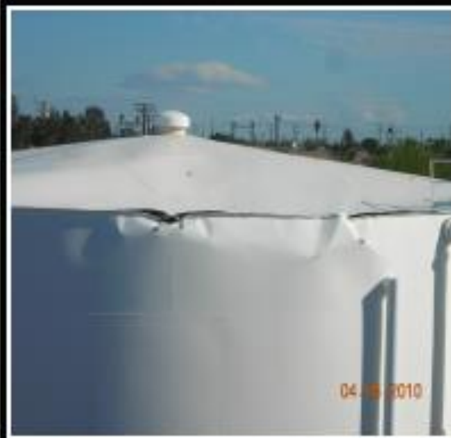
Damage to Roof of Water Tank #3
