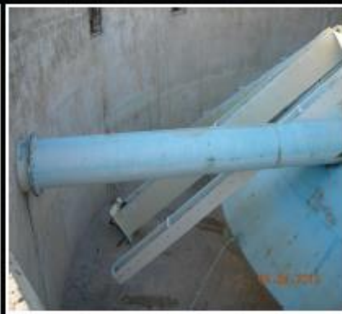
Bent piping in unit 1
