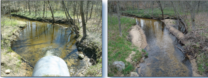
Figure 2. Osborn Creek, looking downstream away from Pierce Road, before (left) and after (right) the culvert was replaced. Downstream sedimentation has declined, allowing the stream to become deeper and narrower.
