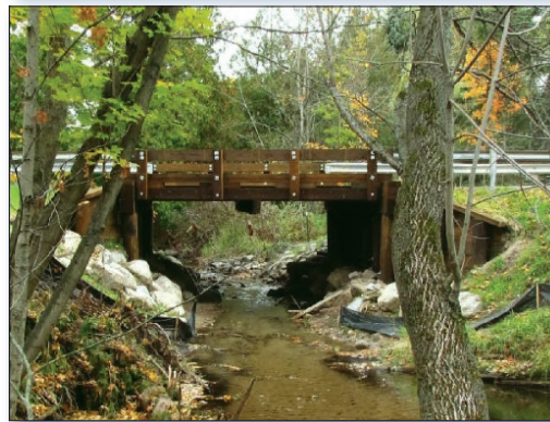
Figure 1. Osborn Creek, looking upstream toward Pierce Road, before (top) and after (bottom) an undersized culvert was replaced with a bridge. Before being replaced, the perched culvert had prevented upstream fish migration. Erosion on either side of the culvert had contributed excess sediment to the creek.
