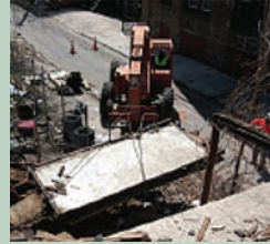
Susquehanna project experimenting with "panelization", where large sections of the row-house are removed intact for disassembly in a staging area.
