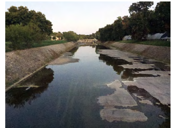
Figure 104 Many of Austin's creeks are channelized like Boggy Creek above. A natural Bouldin Creek is a terrific asset to the city.
