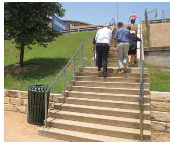
Figure 20 Stairs connect the 20 foot grade change from Statesman Waterfront Park to Congress Avenue at the abutment of the Ann W. Richards Congress Avenue Bridge.
