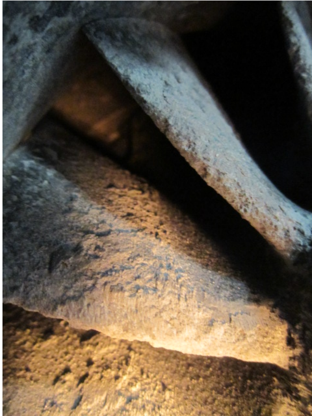
Turbo exhaust blades coated in siloxane after 13,000 hrs
