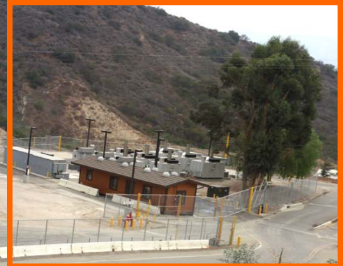
Electric Power Generation
