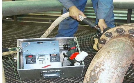
Oil and Gas Systems
