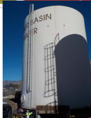
WSWTP 1955 BKW Tank, Weber South Water Treatment Plant, South Ogden, Utah, Weber
