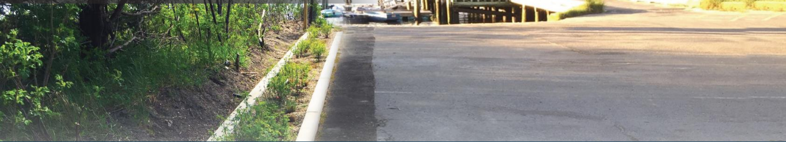
View of the newly installed bioretention swale at the Cotuit Town Dock (Oyster Place) parking lot
